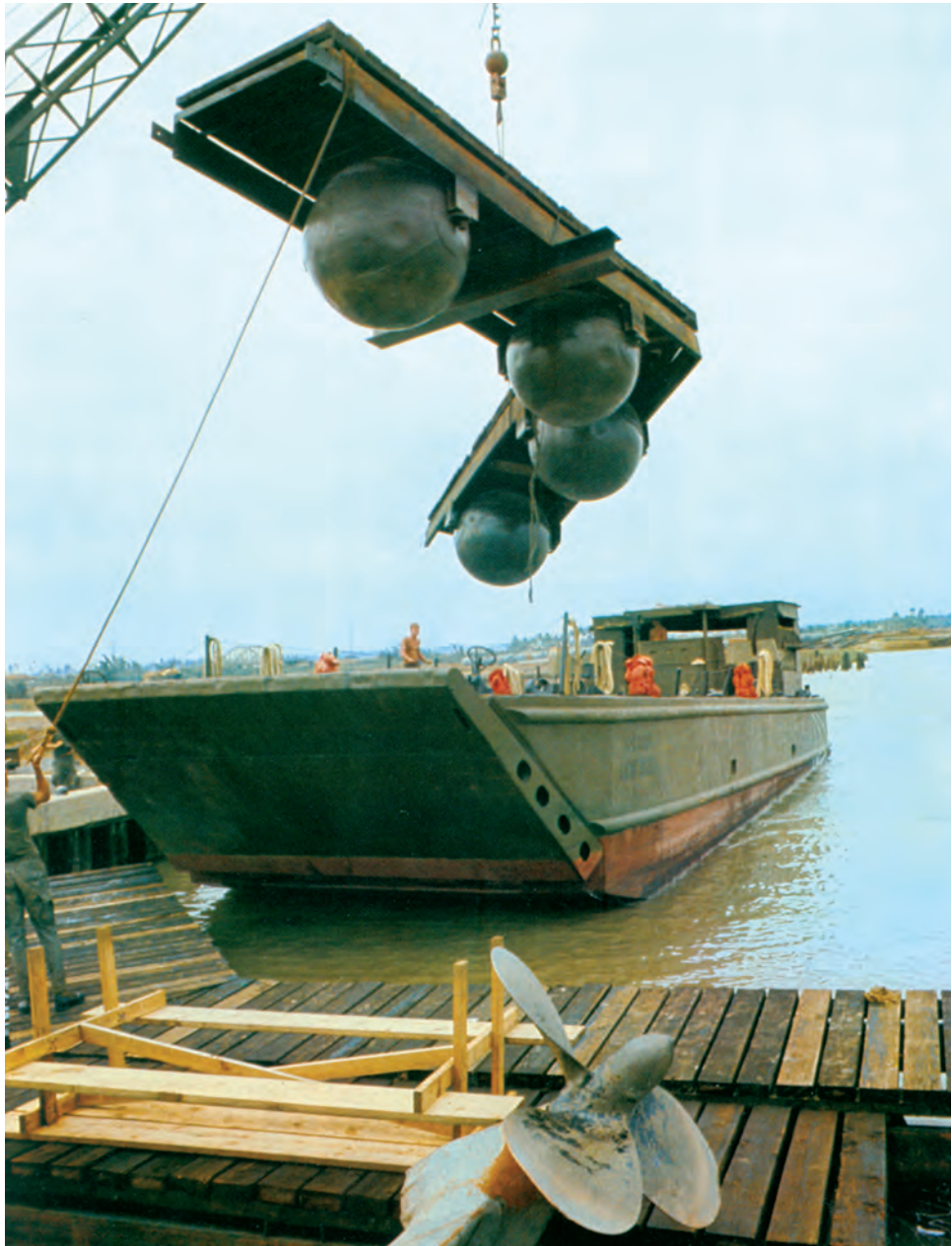
Floating balls being readied for installation at the Phu Cuong Bridge pier protection system
